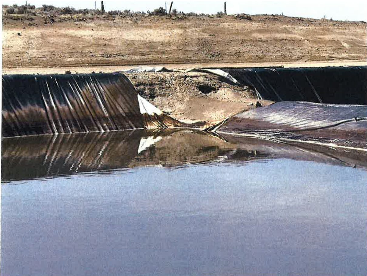
north edge of reserve pit, looking southwest, zoomed in at liner tear
